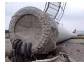
Collapsed due to foundation destruction
